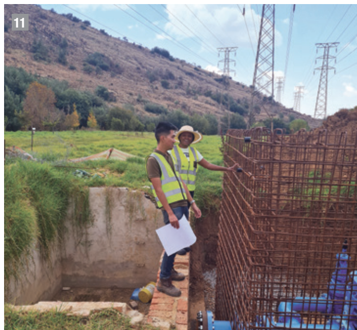
FIGURE 11: Phathi Masimirembwa with Malcolm Low, reviewing reinforcement for a valve chamber on the bulk water pipeline in Linksfield, in preparation for casting concrete
