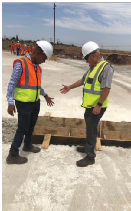
Figure 9: Mentor Ken Bromfield and candidate Aluwani Mudau inspecting reinforcement of a reservoir deck in Jane Furse
