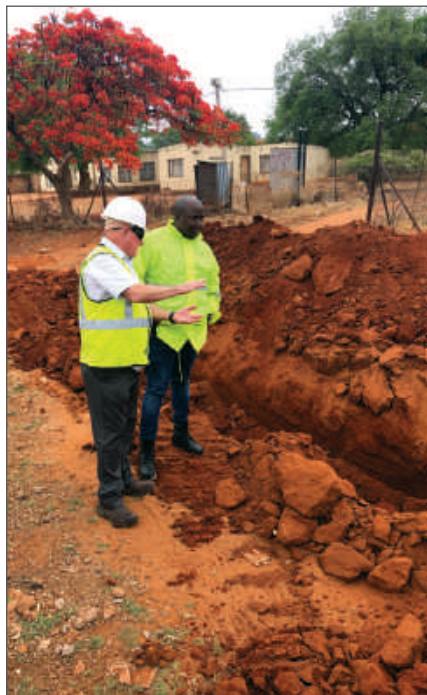
Figure 7: Mentor Ken Bromfield and candidate Christopher Mahlaule inspecting excavations on a water reticulation project in Burgersfort
