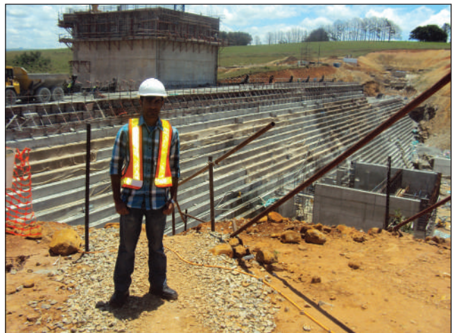
Figure 3: Dhiresh Dhewki, intern at eThekweni municipality inspecting the construction phase of a new dam
