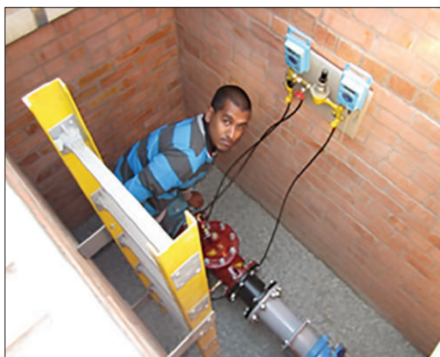
Figure 2: Nishkar Somai , an intern at eThekweni, fixing snags in a pressure reducing valve chamber
